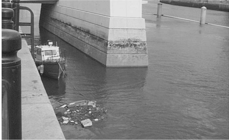
Figure 4. Problems with the vessel collision protection system
